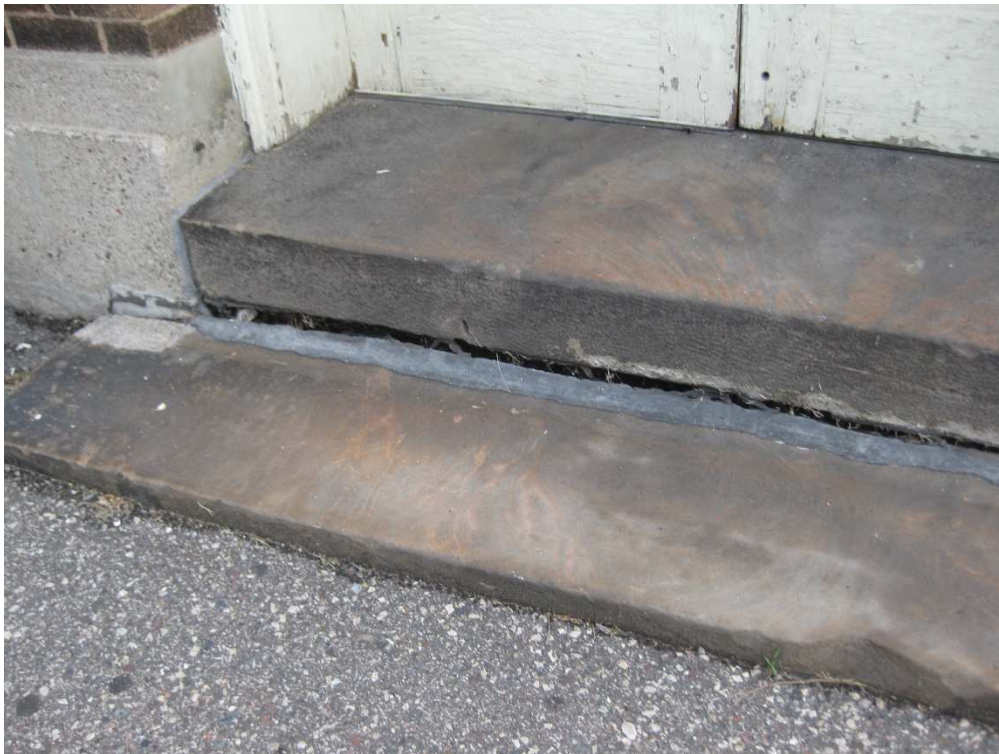
Photo 12 - West elevation - southern door stoop settlement
