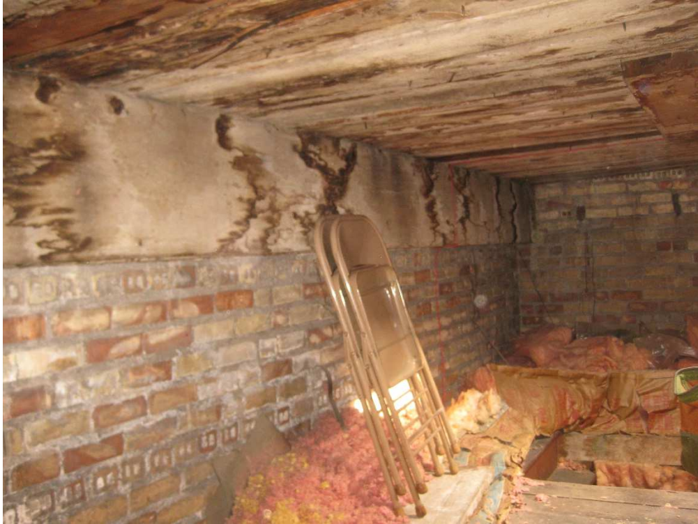
Photo 1 - Roof framing - water stains
