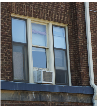
Window air conditioner unit at south side of first floor apartment on west facade.
