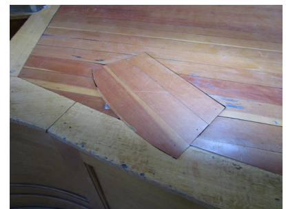
Floor section at the edge of the stage where lights were originally located.
