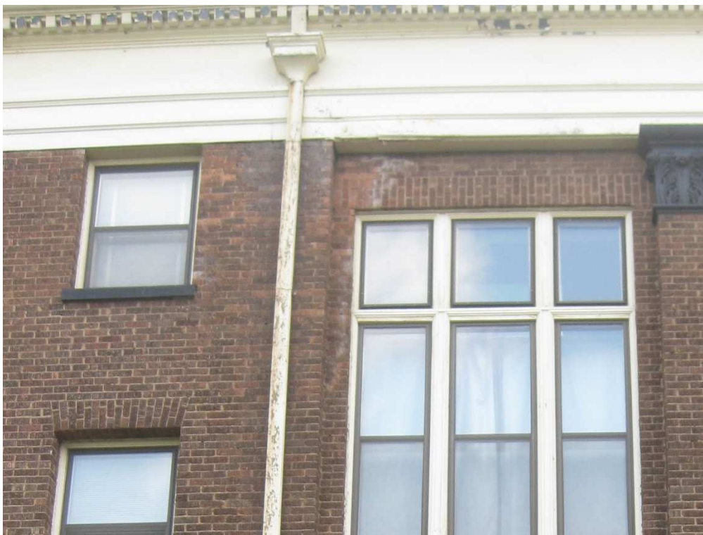
Photo 10 - West elevation showing deterioration at top of wall near downspout
