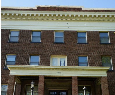
North porch cornice showing deterioration and missing balustrade.
