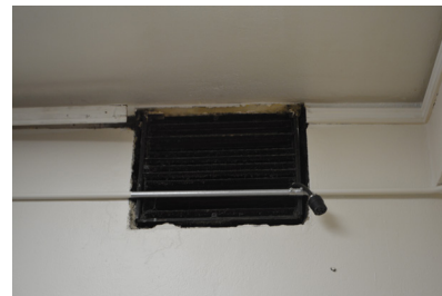
Missing vent cover in Card Room.
