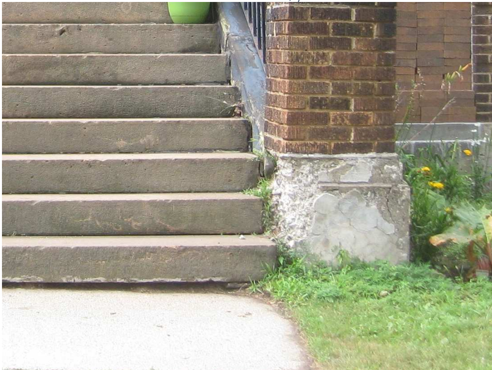
Photo 14 - Front stairs - end post deterioration and settlement of sidewalk
