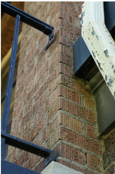
Metal guard rail that has become detached from the brick masonry.
