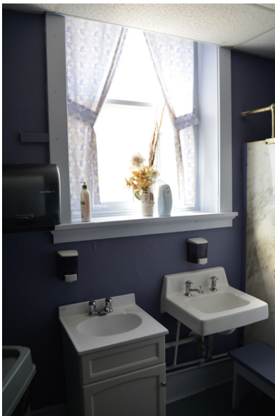
Sinks in the women's toilet room that are not compliant with ADA standards.
