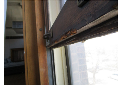
Rail of the lower sash on a window in the Assembly Hall.
