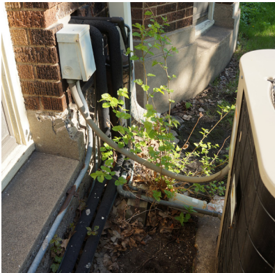
Concrete cracking near pipe penetrations on the east facade.
