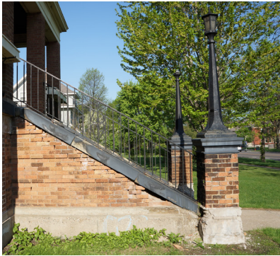
Masonry deterioration at the east wing wall of the porch stairs.
