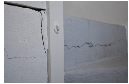
Cracks in concrete adjacent to guardrail in East Dressing Room.
