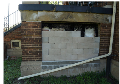
Downspout at the west side of the north porch that dumps water too close to the building.
