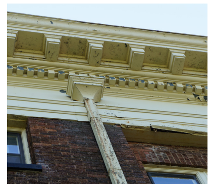
Black stains and efflorescence on the brick surrounding the north downspout on the west elevation.
