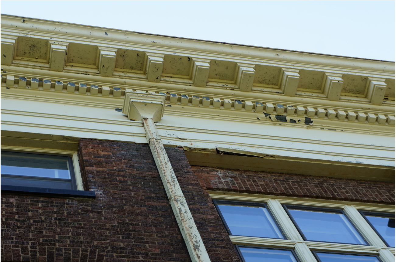
North downspout on the west facade of the building, showing corrosion, loose seams, peeling paint, and damage to the surrounding masonry.
