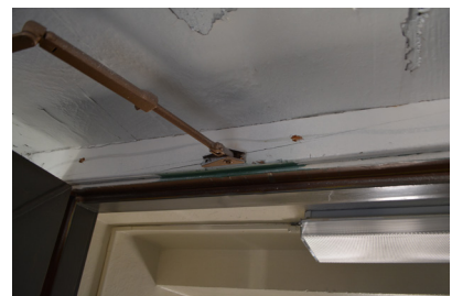
Cracks in wood casing above door.
