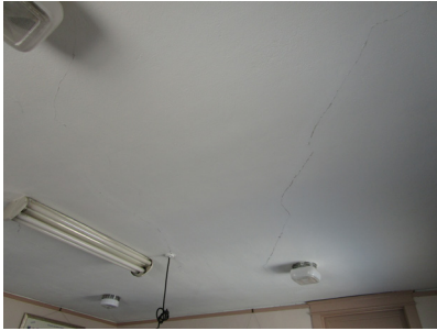
Cracks in plaster ceiling of the Printing Office.
