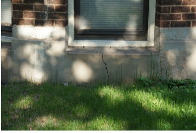
Vertical crack in the concrete below the center opening in the bow window.
