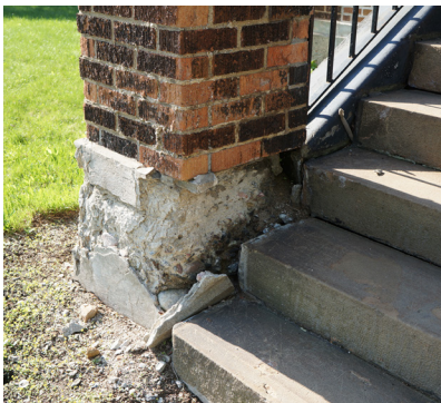
Concrete deterioration at the base of the east post of the porch stairs.
