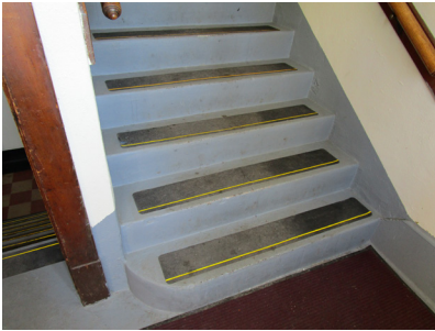
Adhesive treads on the back stairs between the basement and the first floor.
