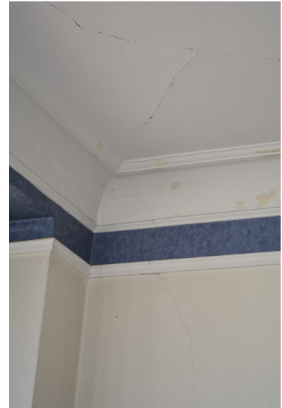
Cracks in plaster wall through the crown molding and ceiling in the Parlor.
