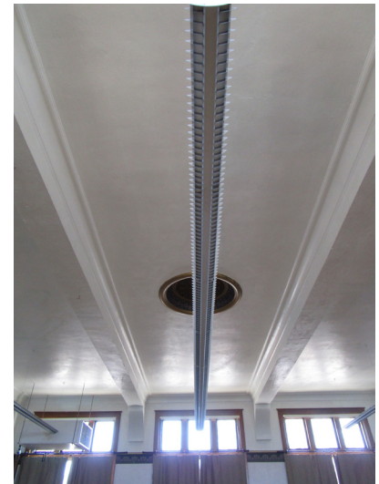
Ceiling in the assembly hall, photograph showing circular vent, plastered wood beams, and florescent lights.
