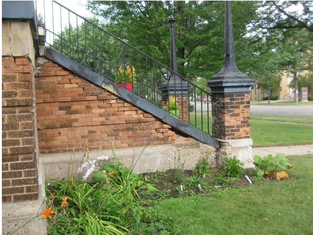
Photo 15 - Front stairs - sidewall deterioration
