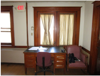
Desk and chair blocking doors from lobby to balcony.
