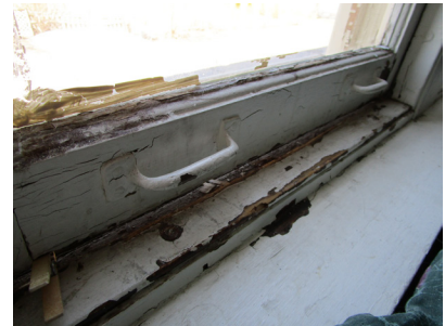
Condition of bottom of window and sill in the bedroom.
