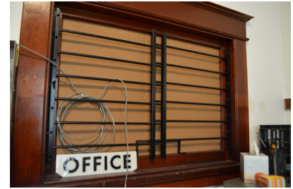
Interior window between the committee room and the passage to the men's toilet room.
