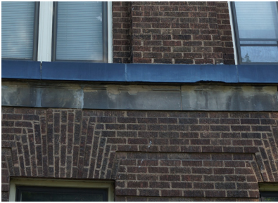
Chip out of cast stone water table on east facade.
