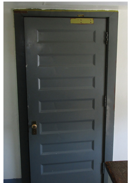
Missing closer at first floor door from back stair.
