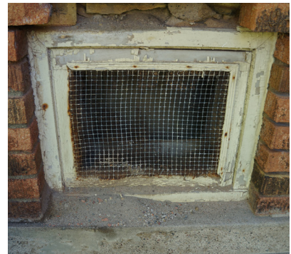
Opening in west wing wall of porch stairs.
