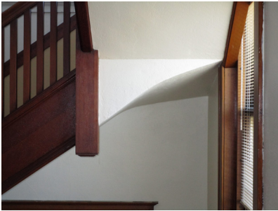
Underside of the last front stair landing before the third floor. Photo taken from the second level.
