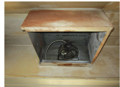
Vent in kitchen.
