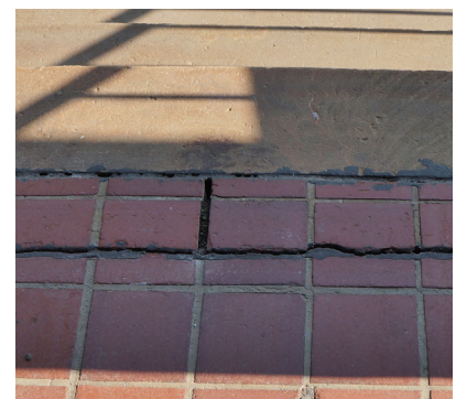
Crack through quarry tiles at north edge of porch.
