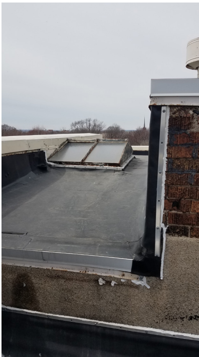
The elevated portion of the roof over the stage has several condition issues, including the membrane itself, the parapet coping, and the skylight.
