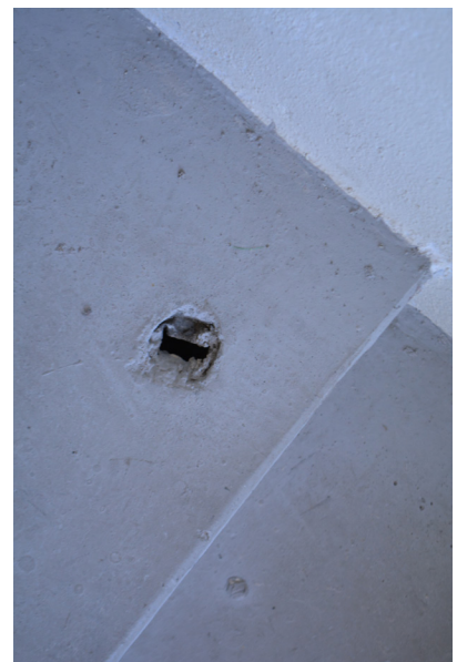
Hole in concrete at top of stairs in East Dressing Room.
