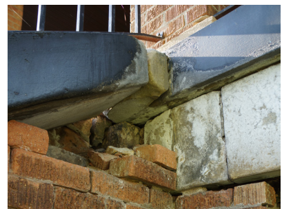
Missing brick below the cast stone cap at the top of the porch stairs' west wing wall.
