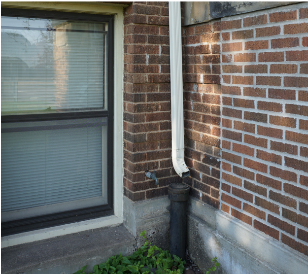
Short downspout on the east side of the porch.
