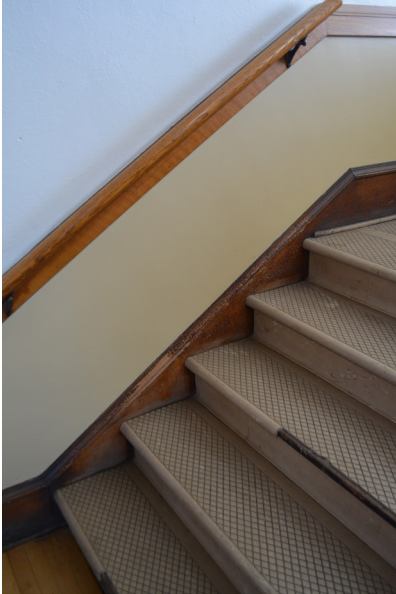
Photograph showing chips in nosing of front stair, deteriorated finish at wall stringer trim, and inadequate handrail extension.
