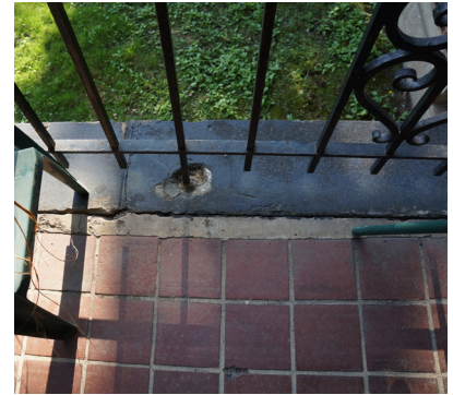
Large grout joint between cast stone and quarry tile floor at east edge of the porch.
