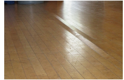
Buckling pieces of wood floor in the Assembly Hall.
