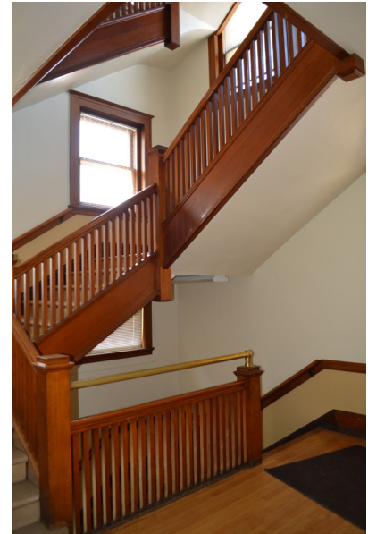
Photograph of front stair at first floor lobby. The bottom of the wood guardrail is stained.
