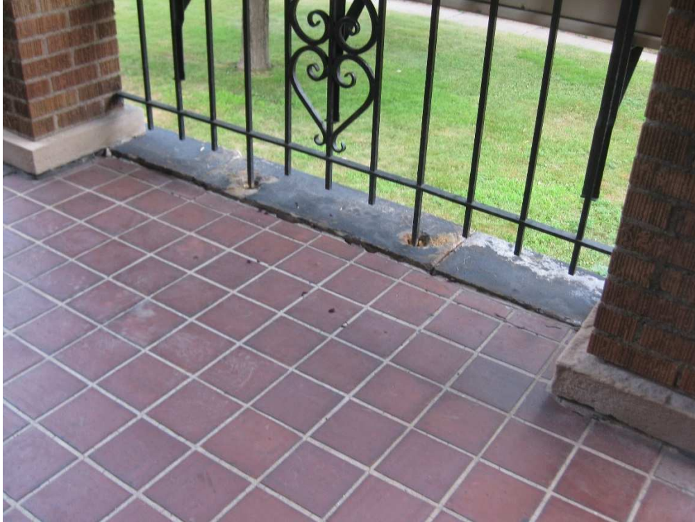
Photo 17 - Front porch - railing attachment damage
