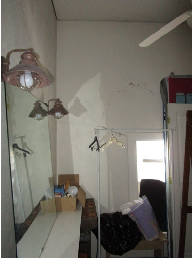
Paint failure and plaster cracks above window in West Dressing Room.
