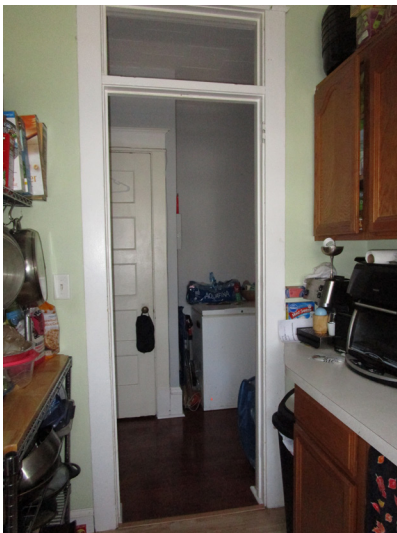
Door frame to kitchen without door.
