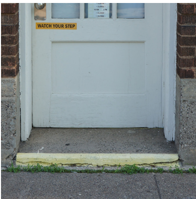
Horizontal crack in concrete in south door sill.
