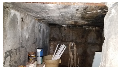
Moisture issues in the Boiler Room.
