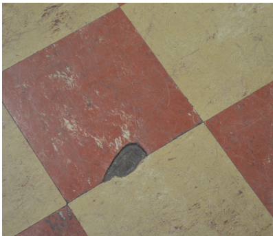
Chipped vinyl asbestos floor tile in the Card Room.
