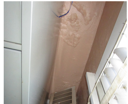
Bumps in paint and plaster in the small office on the third floor.
