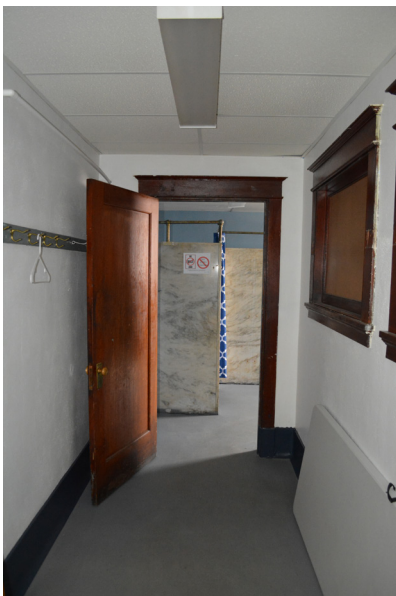
Passage showing boarded up interior windows between Committee Room and Men's Toilet Room.
