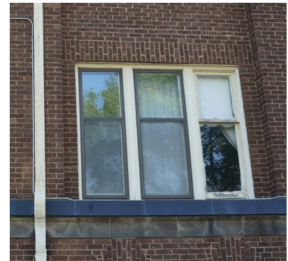
Missing storm window near north side of west facade at the first floor.
