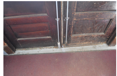
Missing cover at the bottom of the west entry door panic bars.
