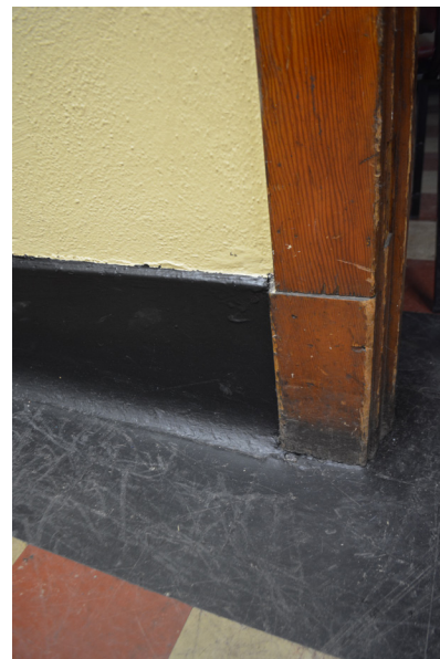
Discolored bottom of door casing in the basement Card Room.
