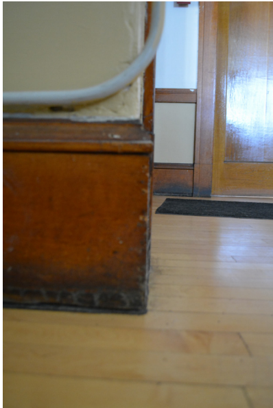
Discolored baseboard in first floor lobby.
