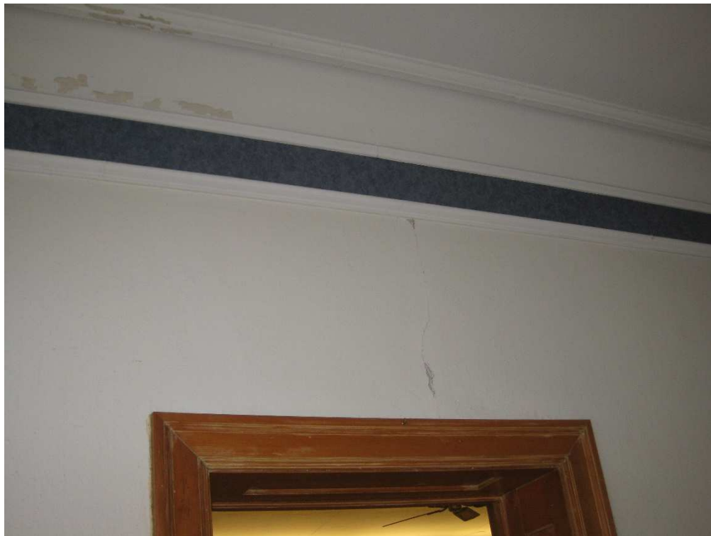
Photo 6 - Ladies Parlor - crack above door in south wall
