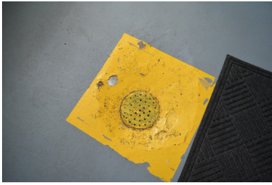
Floor drain in Women's Toilet Room.
