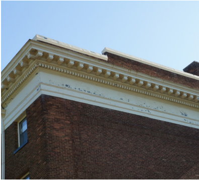
Black stains and efflorescence on the brick beneath entablature on south side of building.
