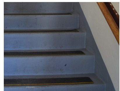
Adhesive treads on stairs between the exterior door and the landing to the apartment.
