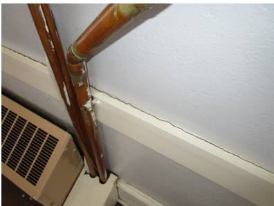
Paint cracks around boards that are pulling away in the third floor hallway.
