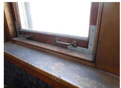
Window in the Assembly Hall which has been stabilized with metal brackets.
