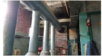
Equipment in boiler room, photograph facing south.
