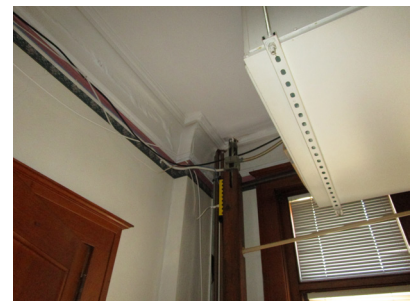
HVAC unit, exposed wires, pipes, and damaged paint on crown molding at northeast corner of Social Hall.
