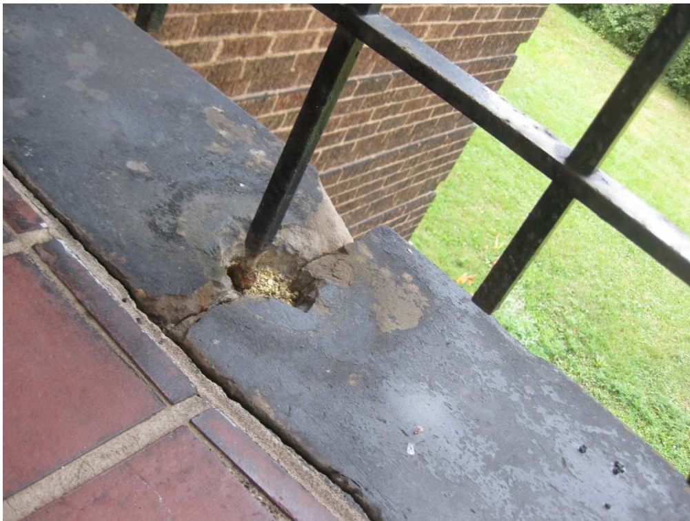
Photo 18 - Front porch - railing post deterioration
