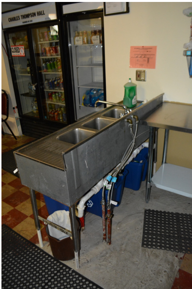
Condition of floor beneath the kitchen sink.
