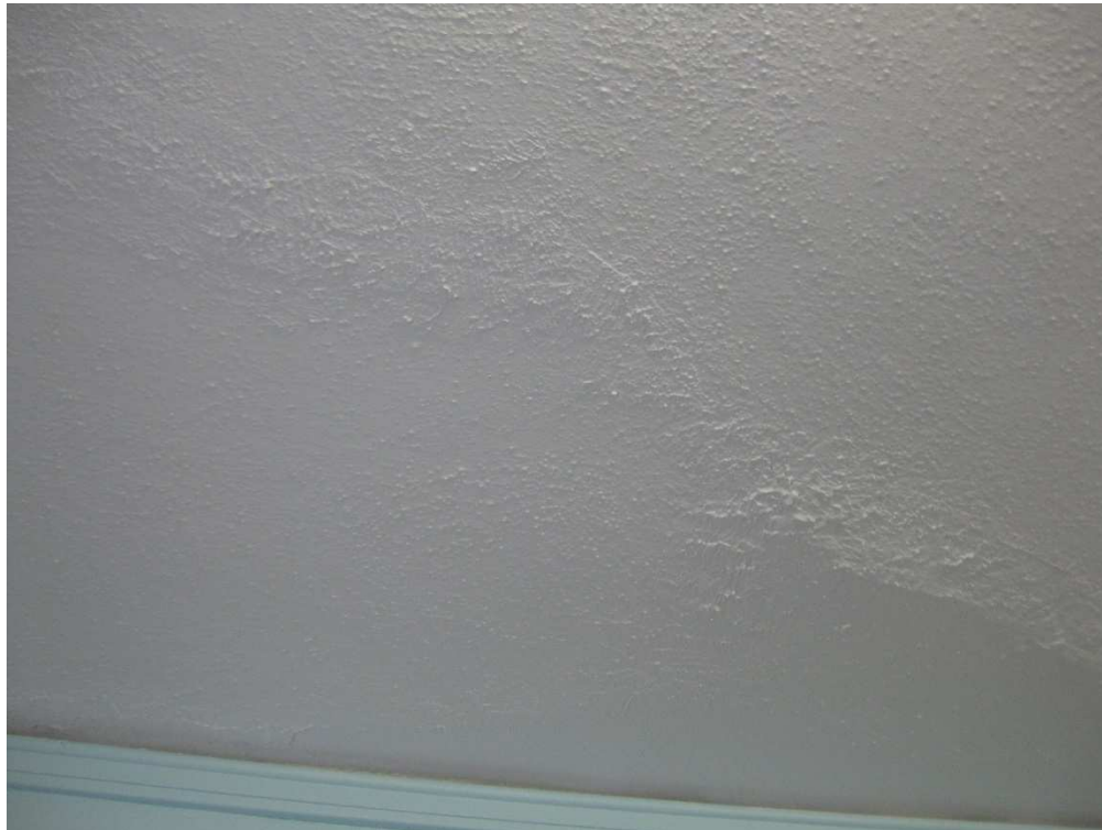
Photo 8 - Ladies Parlor ceiling - previous crack that has been patched
